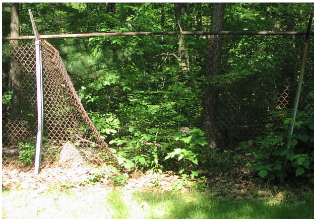
Existing break in chain link fence.
