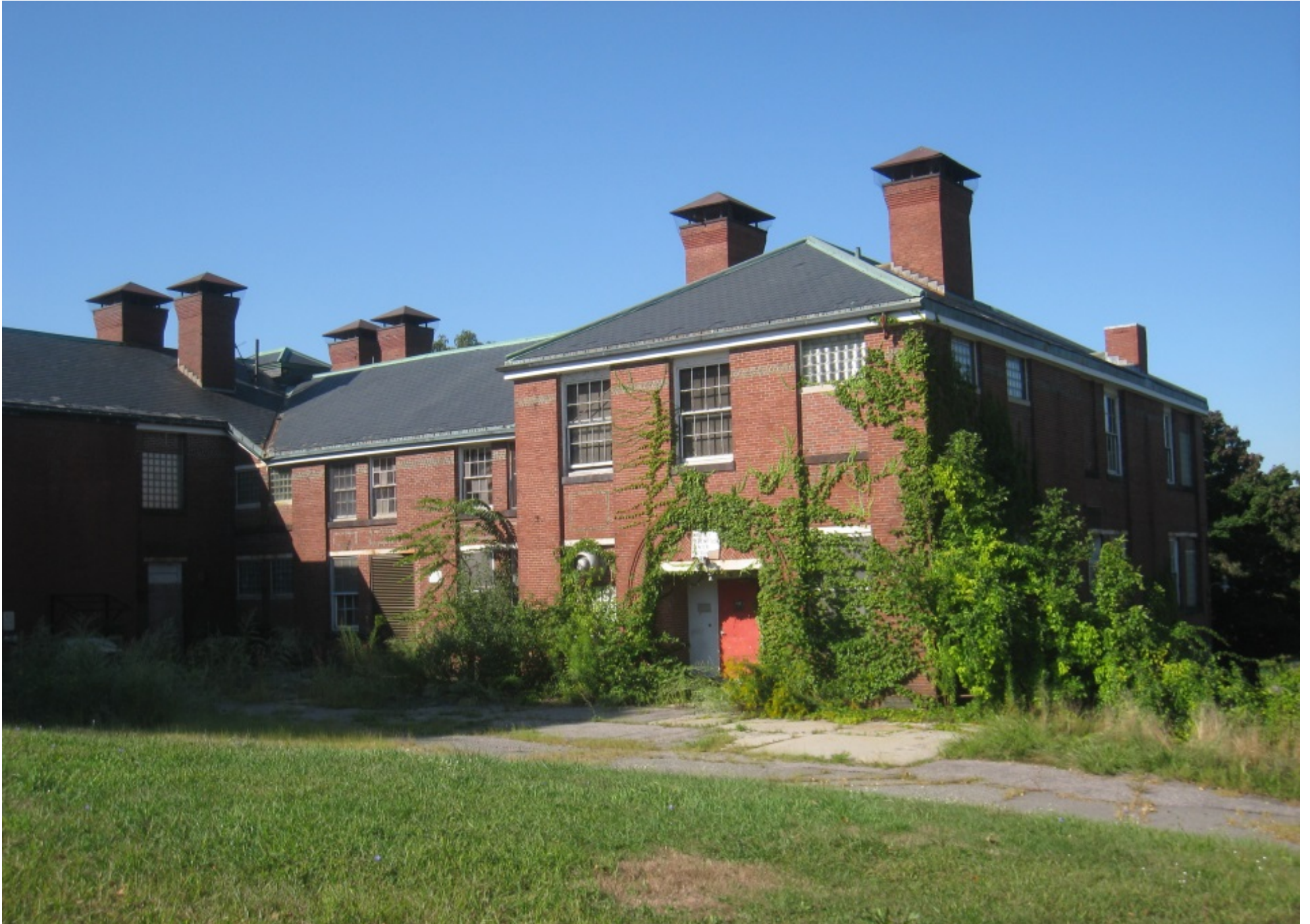
Figure 4: One of the buildings at Fernald. The buildings are in various stages of deterioration. Source: Daderot.
